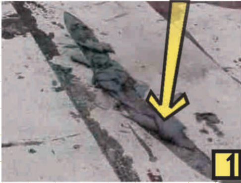
Blisters on existing roof surface
