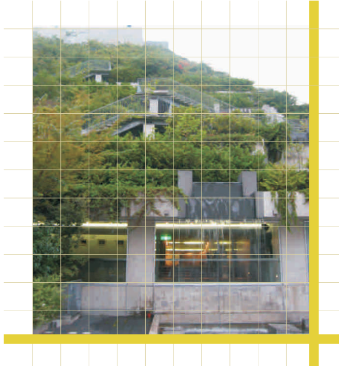
Figure 25 Green Vegetative Roof – Intensive Roof System
