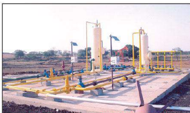
CBM Gas / Water Separation Facilities of RIL
