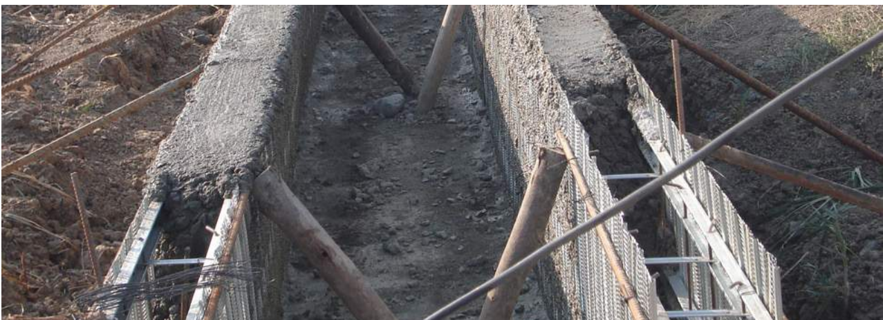
Figure 26: Photographs of the assembly of 'Coffor' panels without insulation (first) and filled with concrete on-site (second). Source: (Coffor Construction Company LLD, n.d.)
