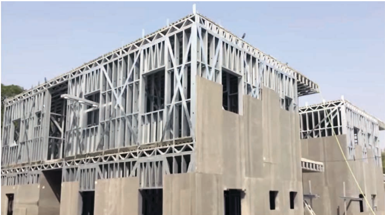
Figure 13: Photograph showing walls and floor plates of LGFSS assembled at a site.
