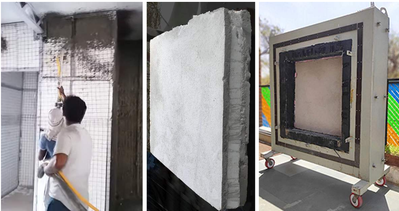
Figure 20: Example of on-site shotcreting (left), Sample of EPS core panel received from the manufacturer (middle) and EPS core panel fixed into the specimen frame of GHB(right) Source: (left) (BMTPC, 2018a)
