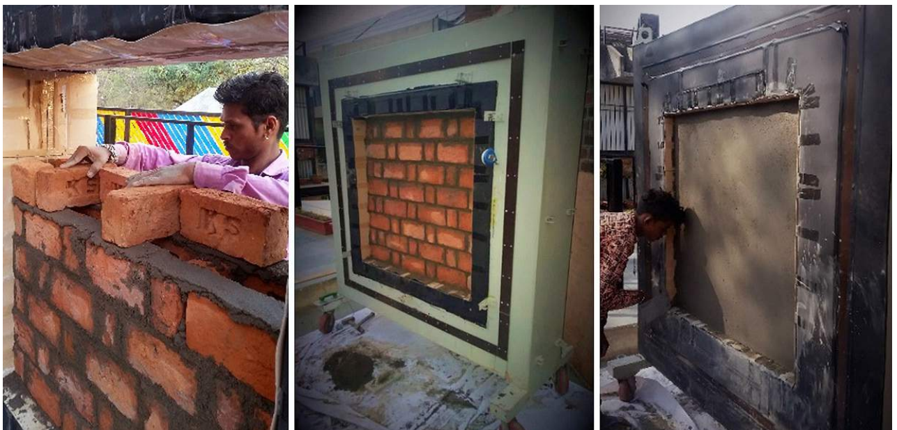
Figure 12: Photograph showing the construction of Rat trap bond wall within the specimen frame of GHB.
