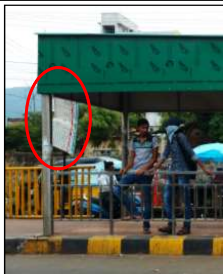
Figure 2: A typical bus stop along the corridor - Highlighting major issues in at the BRT stations
