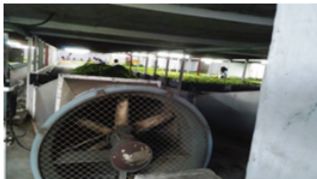
Figure 2. Axial fan attached to withering bed
