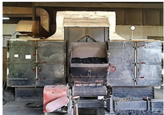
Figure 5. Coal-based hot air generator (HAG) for drying
