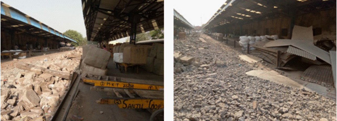
Figure 33: Photographs showing the poor condition of access points for parcel holding/loading areas at the Old Delhi Station (May 1, 2018)
